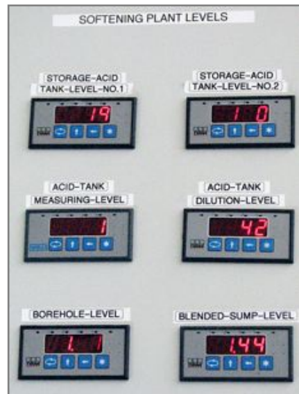
Water softening plant: water level monitoring.
