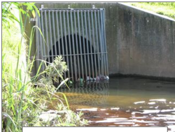
Basin 6: Storm water inlet with entrance covered to prevent children playing inside.
