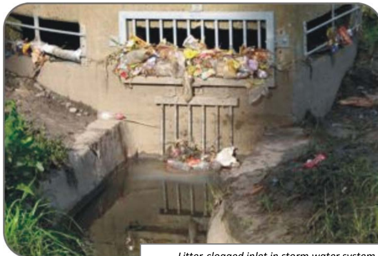
Litter-clogged inlet in storm water system.
