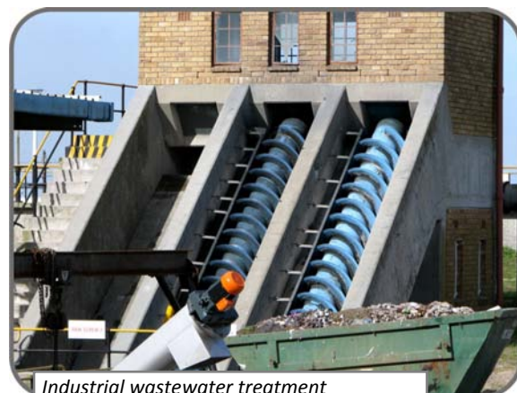
Industrial wastewater treatment works.
