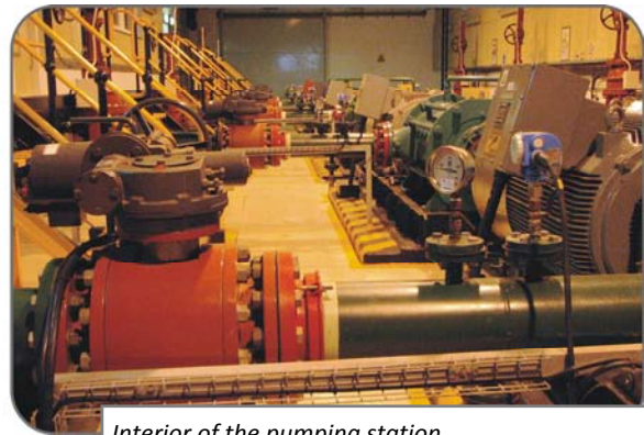
Interior of the pumping station.
