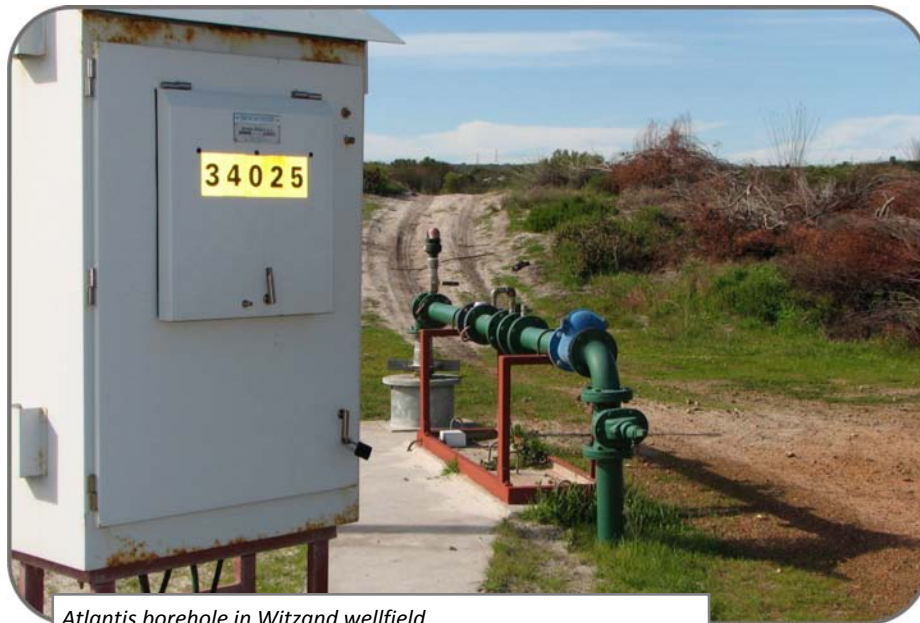
Atlantis borehole in Witzand wellfield.
